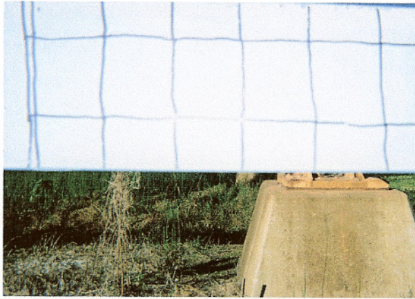
ASTM 610 Rust grade 9 M 714 Scale 10
